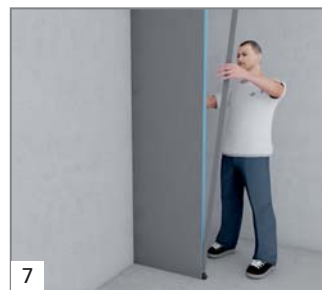
7 Connection of two Moltoromo wall elements makes it necessary to insert the tongue into the groove before the glue has cured. In such case, the bottom of the tongue rests on the installation block.
