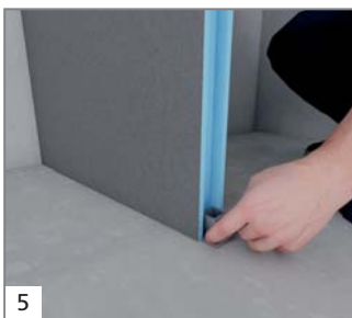
5 An installation block is inserted on the floor to stabilise the Moltoromo wall elements. The installation block is positioned in the specified groove in the wall element.
